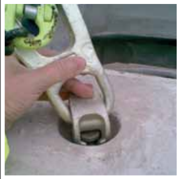
DEHA lifting link Connected to cast in anchor pin on Cover Slab. (In accordance to the manufacturer's guidance specification)
